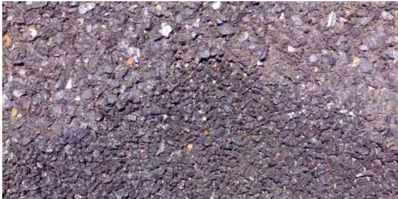
ROADFIX CA Patch - Note how the COLD ASPHALT joins to the edge of the pothole & no priming was required.
