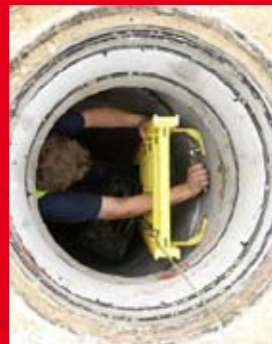
Anchoring ladder in the access chamber
